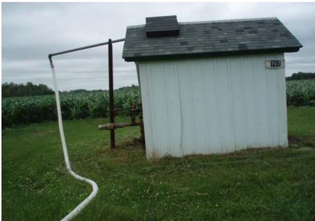
Pump House for Well 207608
