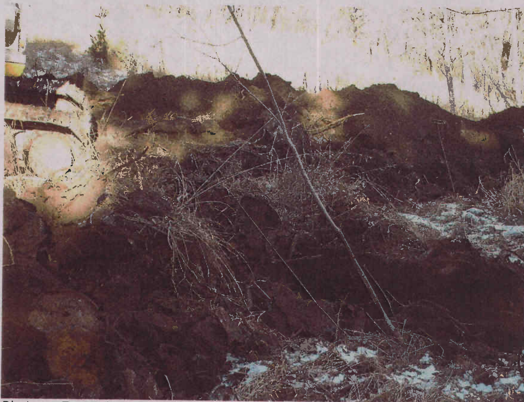
Burn Pit Area. Excavation of test pit BP-TP-10 which confirmed the drum components at this location are surficial.
