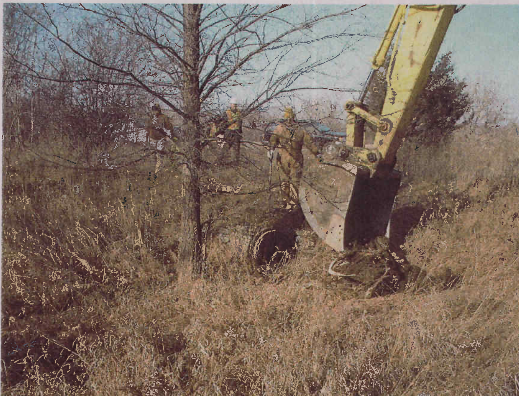
Nitric Acid Plant Area. View of test pit NA-TP-2 which was completed adjacent to the south open end of a wooden drainage culvert that runs under 152 nd Street.
