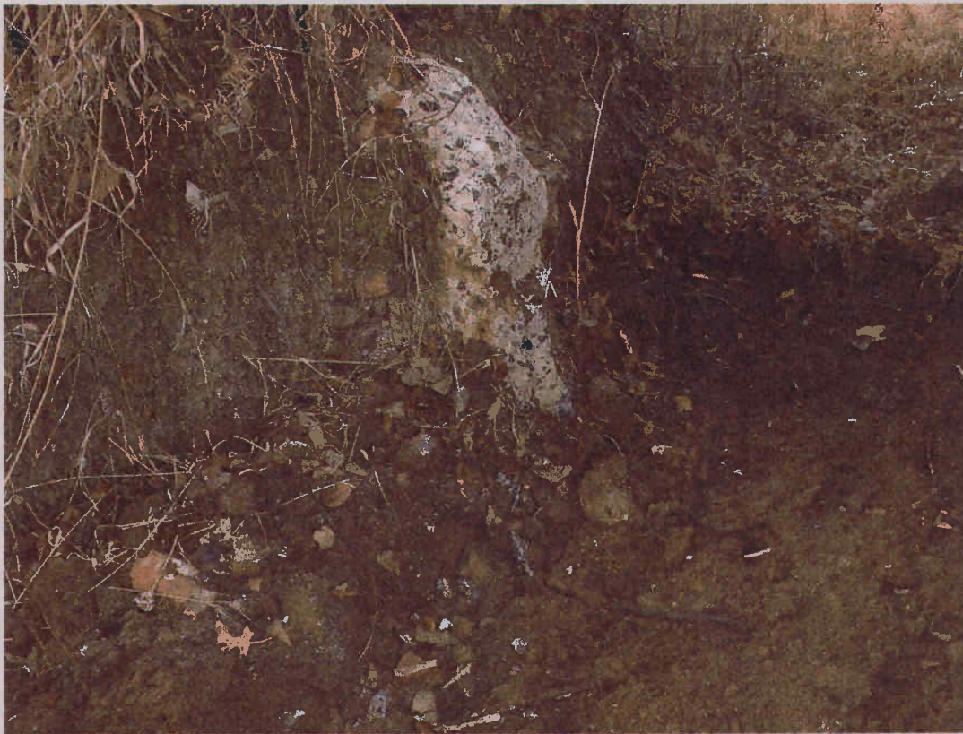
Oleum Plant Area. View of test pit OP-TP-1 showing the base of the sulfur mixing pit which is 2 feet below current grade. The base of the sulfur mixing pit is brick and the walls are constructed of poured concrete.
