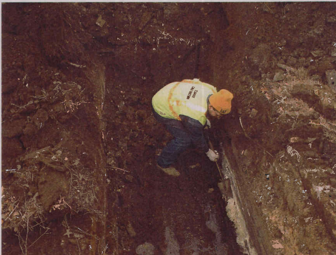
Oleum Plant Area. View of test pit OP-TP-2 showing the base of the sulfur mixing pit. Note the 6 inch layer of sulfur product at the bottom of the mixing pit.
