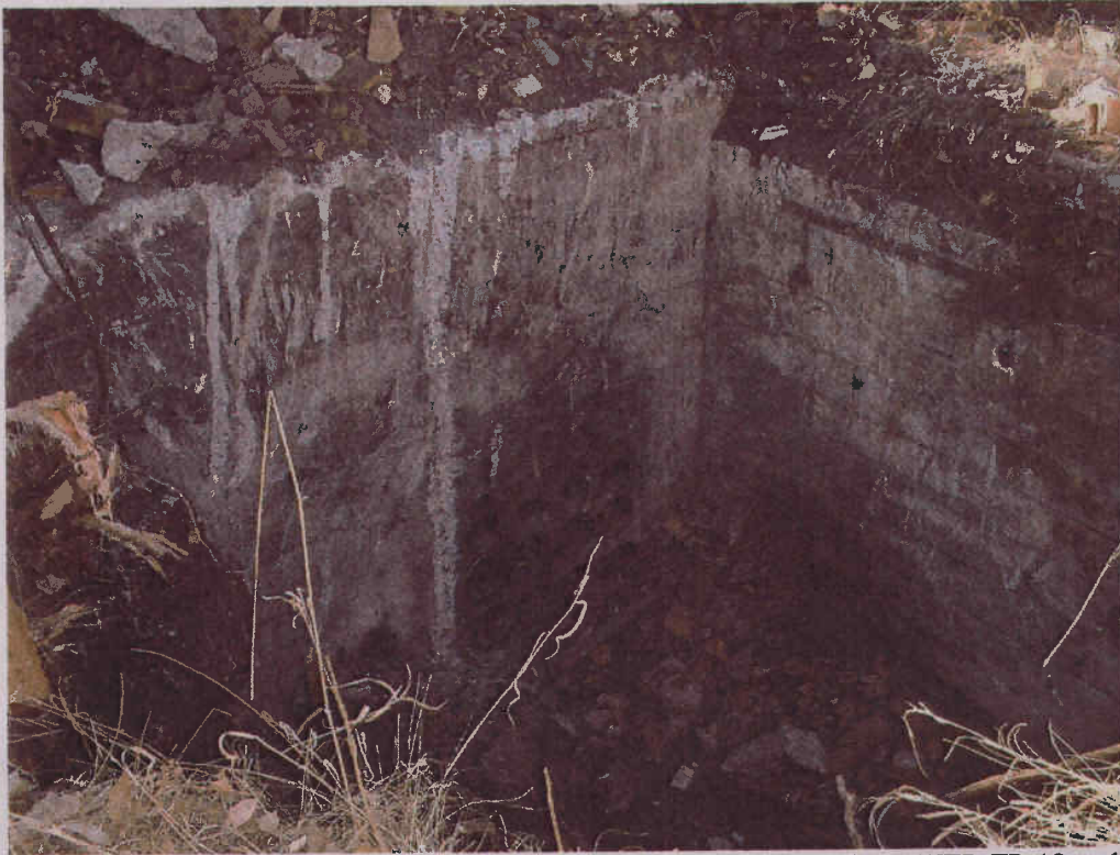
Wastewater Treatment Plant Area by Power Plant A. View of test pit WWTP-TP-12, which was excavated within a subsurface concrete water holding tank. The tank was filled with soil and debris.
