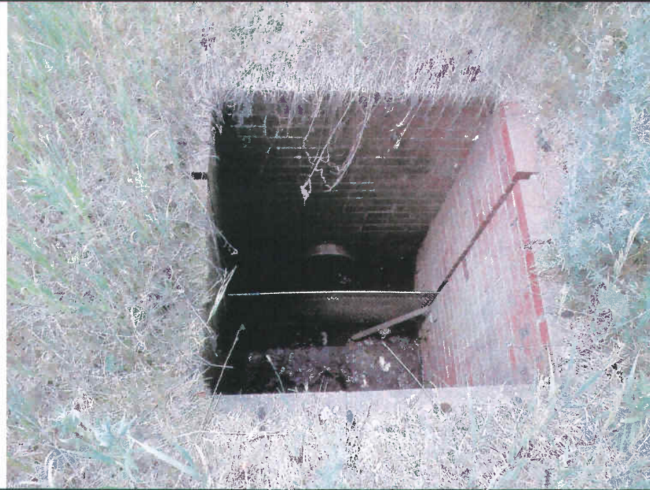
Photo 12: Open sump near building 105-B
