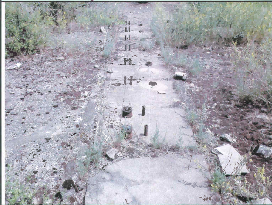
Photo 16: 109-B Conduits in concrete
