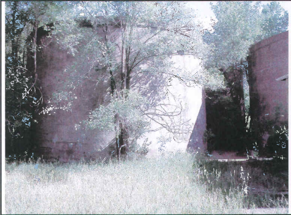
Photo 35: 401-BB1 Power Plant B Precipitators
