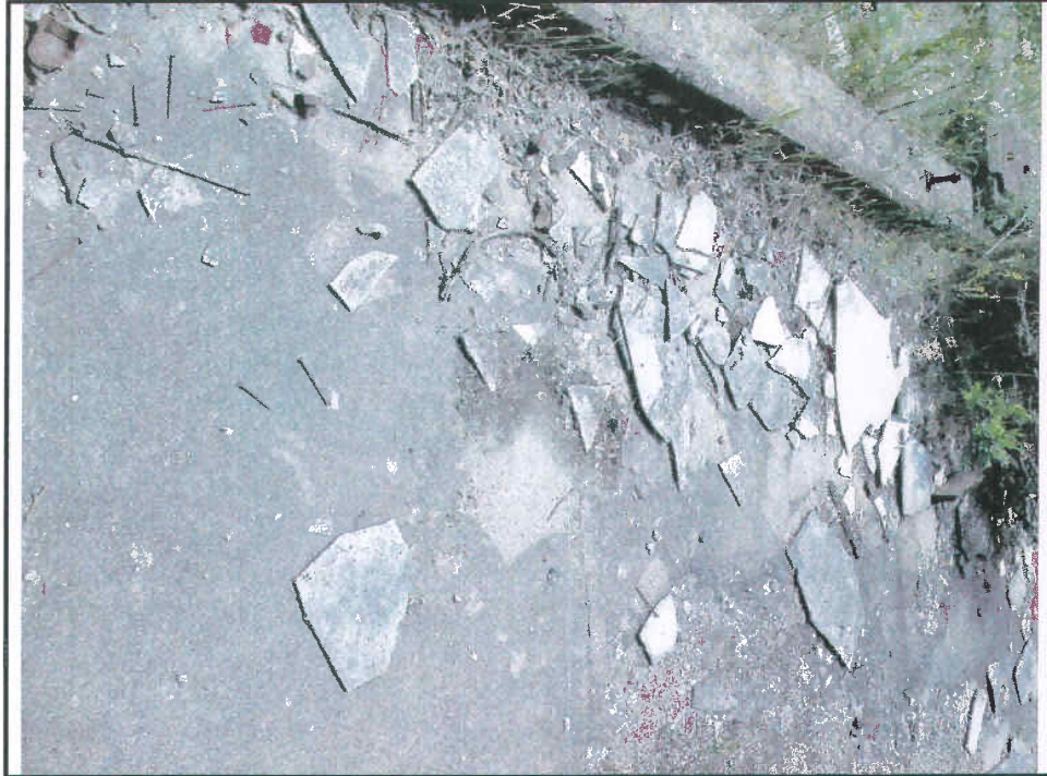
Photo 19: 113-B Potential asbestos containing material (ACM)
