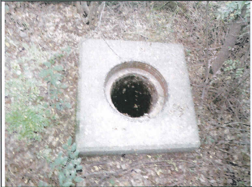
Photo 8: Open Pipe near 105-F
