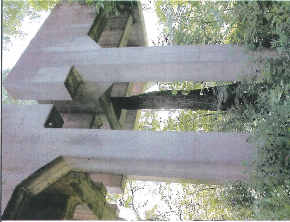
Photo 41: 305-B East Acid Area support structure remnant
