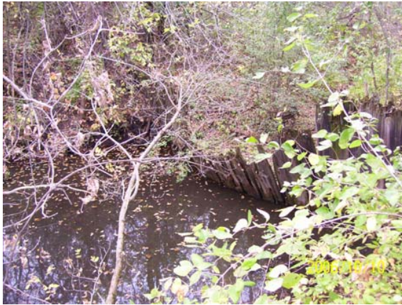
Photo 1. AOC 1. Remnants of gated weir/dam structure at the Southeastern end of the Secondary Settling Basin. (1)
