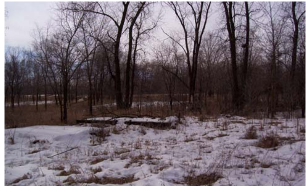
Photo 23. AOC 7D. Two of four of the possible transformer storage pads on the southwest side of Building 401-A. (2)
