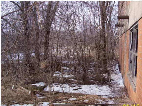
Photo 14. AOC 7A. Possible Transformer storage pad on the south side of Pump House. (2)
