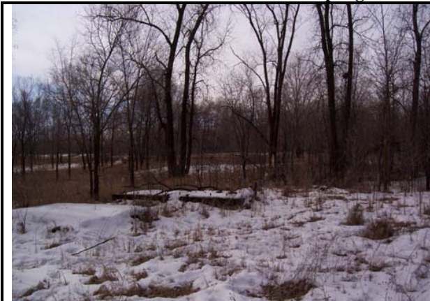
Photo 23. AOC 7D. Two of four of the possible transformer storage pads on the southwest side of Building 401-A. (2)
