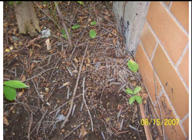
Photo 58. AOC 7A. Discarded small arms practice munitions found next to former transformer pads. (4)
