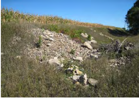
Debris in drainage ditch. This drainage is part of AOC 3-DA1 investigated in Army FSI.
