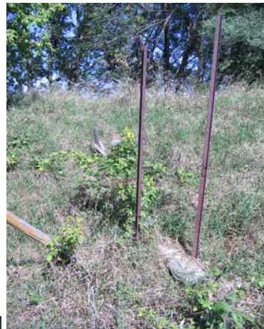
Four inch pipe daylighting in west side of berm into west basin.
