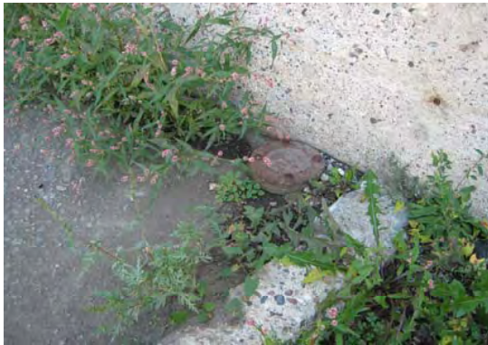
Interior drain gutter and French drain/sump (also known as dry well) in corner of partially demolished DNT storage bunker.
