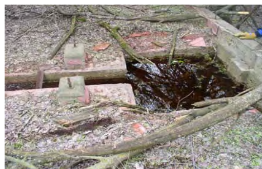
Bldg 237-G Sump & French Drain
