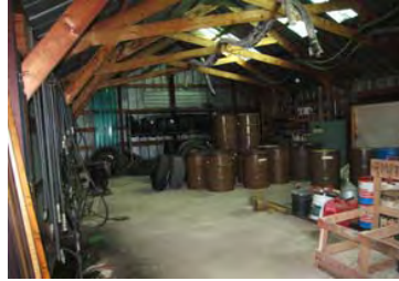
Petroleum storage inside Building 611. Note staining along left edge of floor slab.
