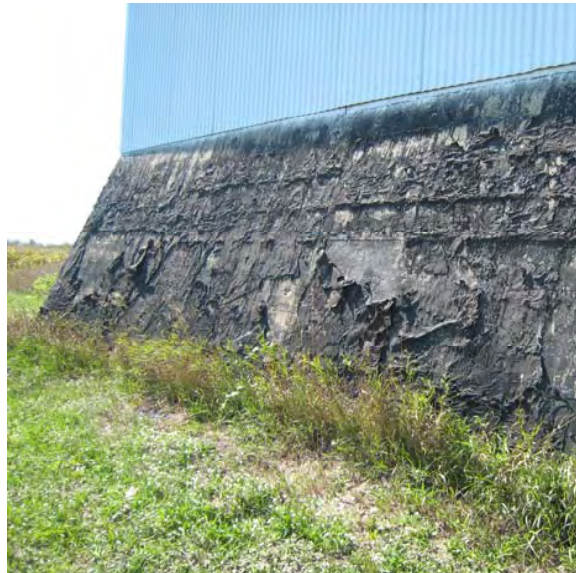
Remnant tar coating on exterior walls of DNT bunkers.
