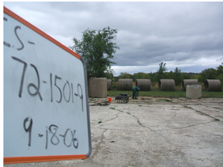
Building 1501-9, facing north, location of concrete sample 72 taken on the concrete building pad.
