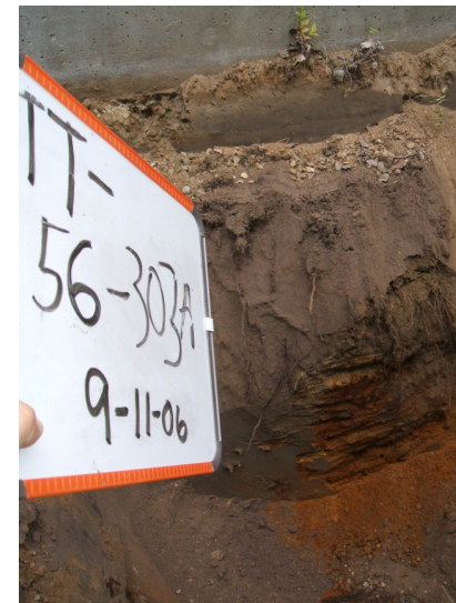
9/11/06: orange stained soil below the eroded concrete wall in test trench 56 located on the west side of the building.
