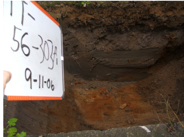
9/21/06: orange stained soil below the eroded concrete wall in test trench 56 located on the west side of the building.
