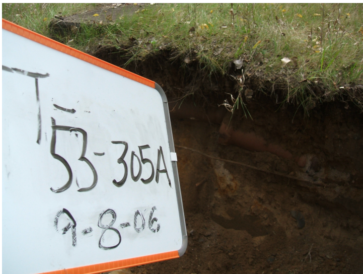
9/8/06: clay pipe discovered in test trench 53 located on west side of the building with stained soil below joints.
