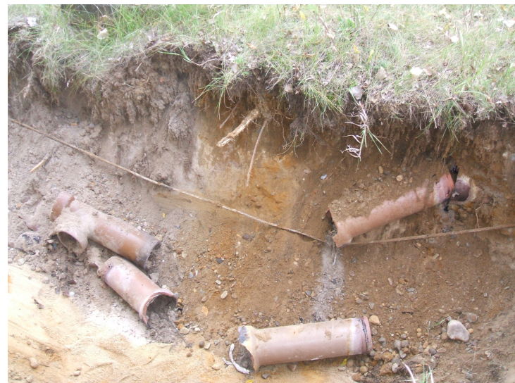
9/8/06: clay pipe discovered in test trench 53 located on west side of the building with stained soil below.
