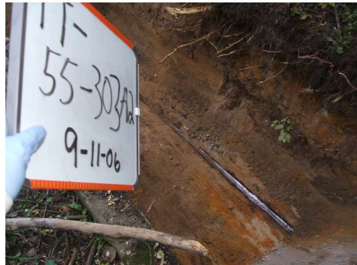
9/11/06: steel pipe discovered in test trench 55 located on southwest building corner with orange stained soil around it.
