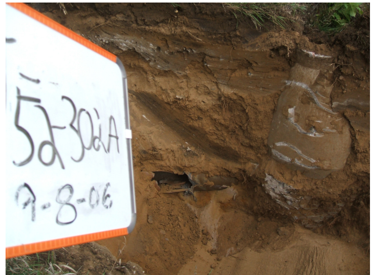
9/8/06: stained soil below pipe discovered in test trench 52 along the east central portion of the former southern building wall.
