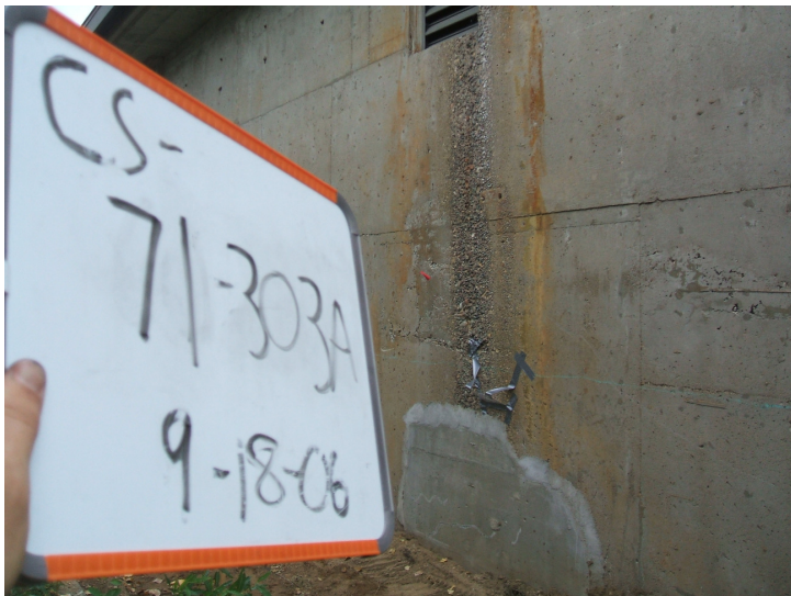
9/18/06: eroded concrete above test trench 56 and location of concrete sample 71 located on west side of the building.
