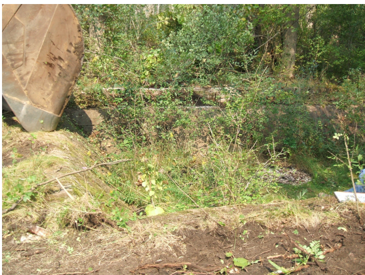
9/6/06: test trench 9 located in the south western portion of the south building wall near a save-all.
