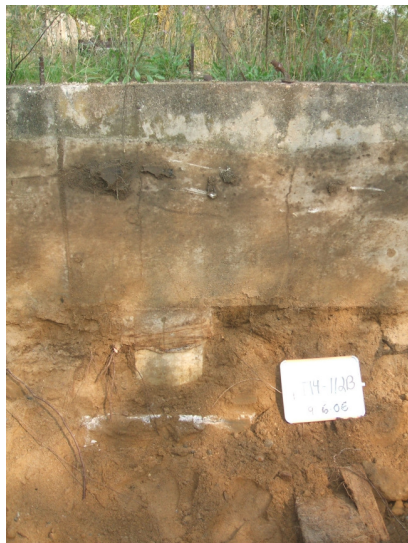
9/6/06: building footing along test trench 14 located along the southern area of the west building wall.
