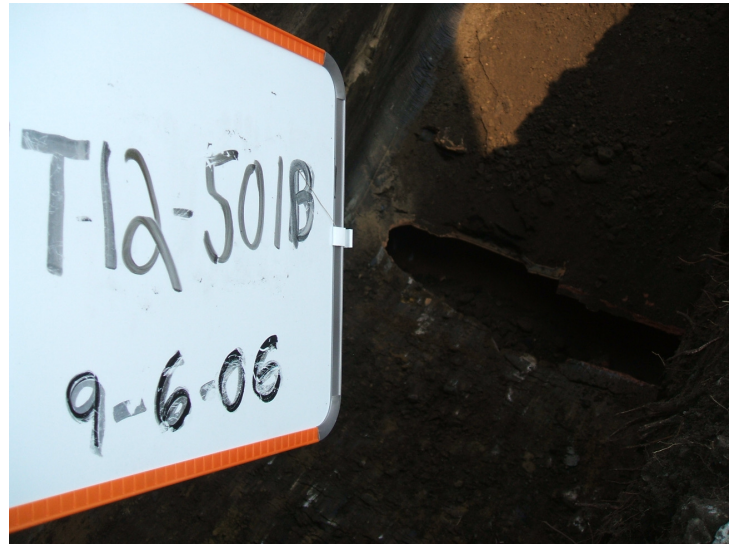
9/6/06: clay pipe discovered in test trench 12 located on the east side of the building.
