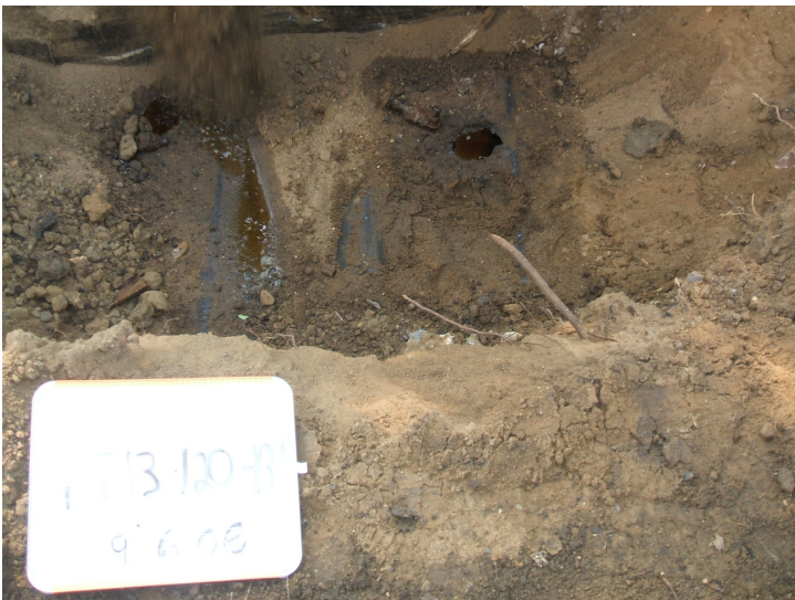
9/6/06: three cast iron pipes discovered in test trench 13 located on the east side of the building.
