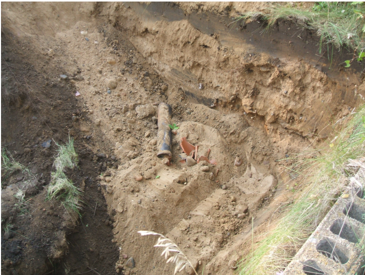
Building 706J, pipes discovered in test trench 15 located on the north side of the building.
