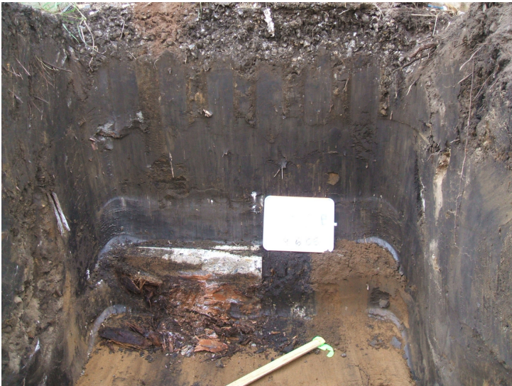
9/6/06: building footing along test trench 12 located on the east side of the building.
