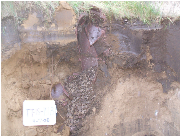
9/7/06: dry well discovered in test trench 18 located on the north side of the building.
