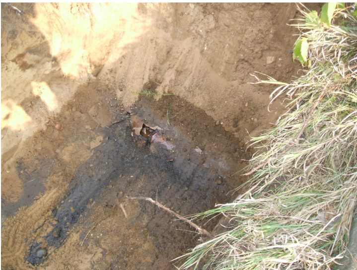
9/6/06: clay pipe discovered in test trench 2 located along the west central part of western building wall.
