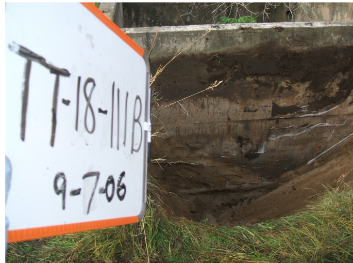
9/7/06: building footing along test trench 18 located on the north side of the building.
