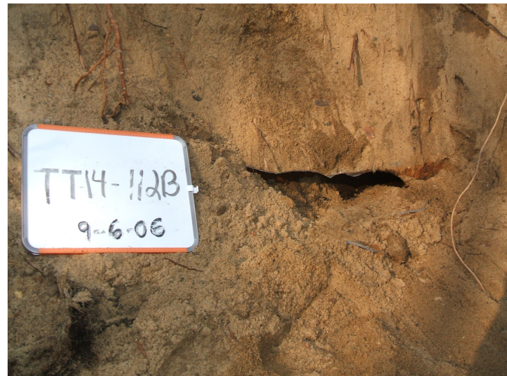
9/6/06: cast iron pipe discovered in test trench 14 located along the southern area of the west building wall.
