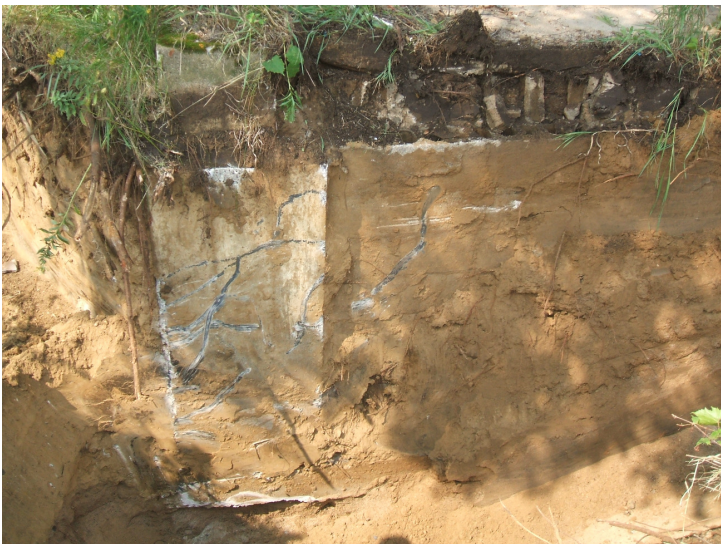
Building 722B, building footing along test trench 6 located on the southeast corner of the building.
