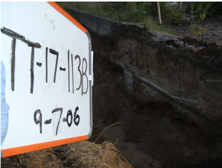
9/7/06: building footing along test trench 17 located along the southern portion of the west building wall.
