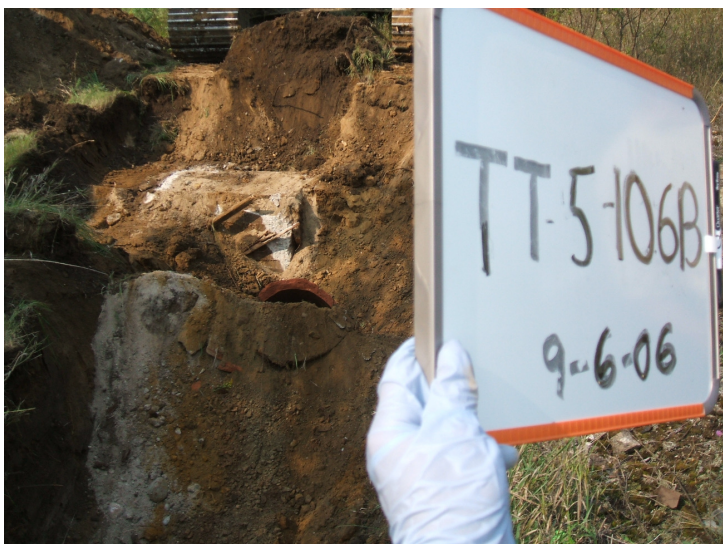
9/6/06: concrete footing and clay pipe in test trench 5 located on south side of the building.
