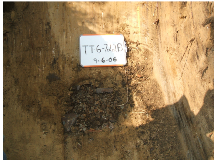
Building 722B, dry well discovered in test trench 6 located on the southeast corner of the building.
