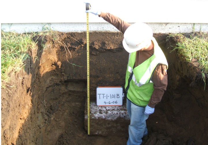
9/6/06: concrete footing in test trench 1, located in the southeast corner of the building.
