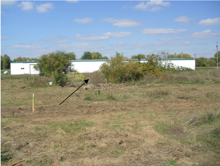
9/20/06: view facing north of concrete building pad location framed out by bushes.
