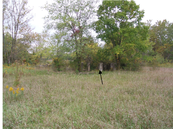
9/21/06: view facing west of concrete supports on building pad. Pad hidden by foliage.
