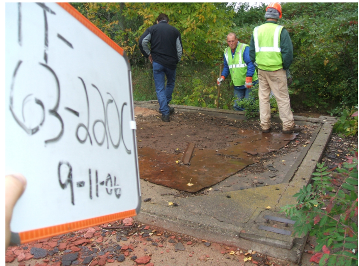
9/11/06: possible ACM red mastic on concrete building pad.
