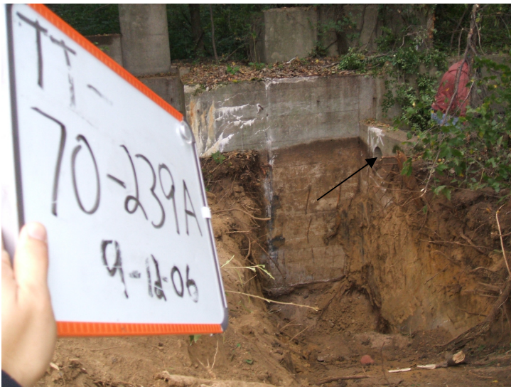
9/12/06: building footing along test trench 70 with view of an overflow drain located on the south side of the building.
