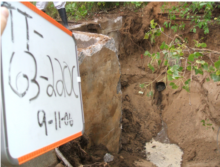
9/11/06: pipe discovered and concrete footing along test trench 63 located on the southeast corner of the building.
