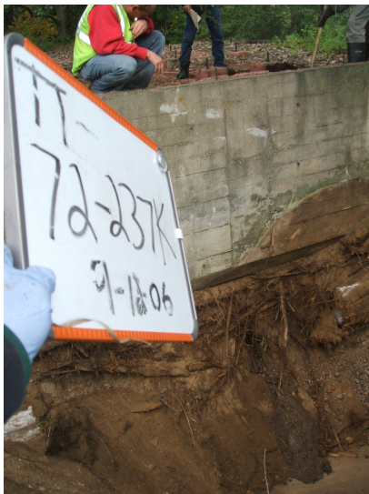
9/12/06: building footing and pipe along test trench 72 located on the southeast corner of the building.
