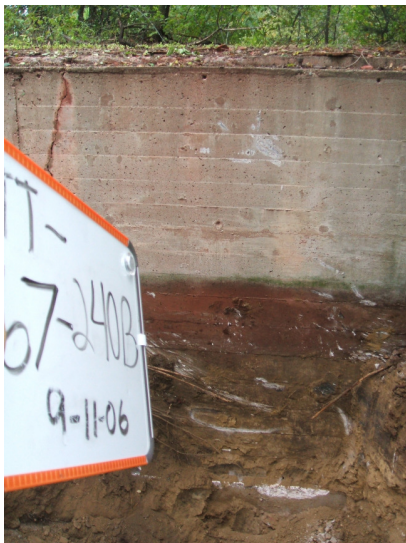
9/11/06: building footing along test trench 67 with red staining from the red mastic on building slab located on the south side of the building.
