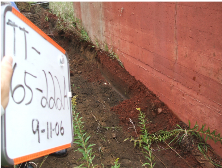
9/11/06: red mastic on soil at test trench 65 located on the south side of the building. Red staining from the flooring mastic on footing wall.
