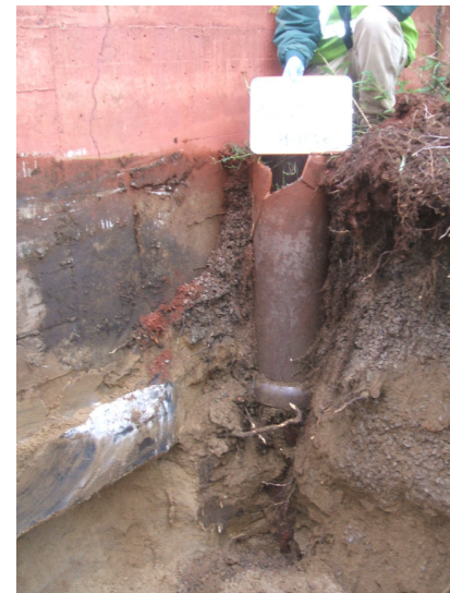
9/11/06: building footing and dry well at test trench 65 located on the south side of the building.
