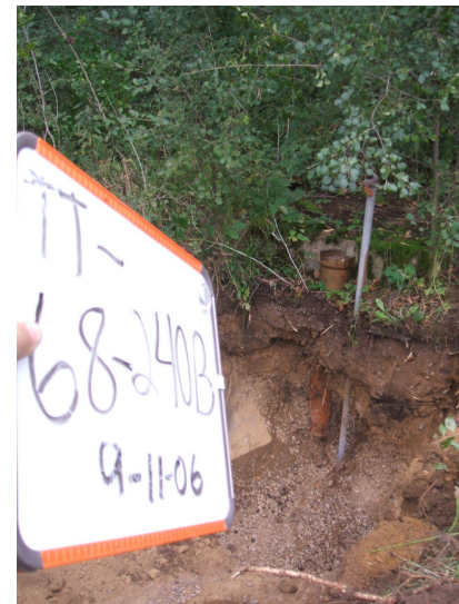
9/11/06: dry well discovered in test trench 68 located just east of the east building wall..
