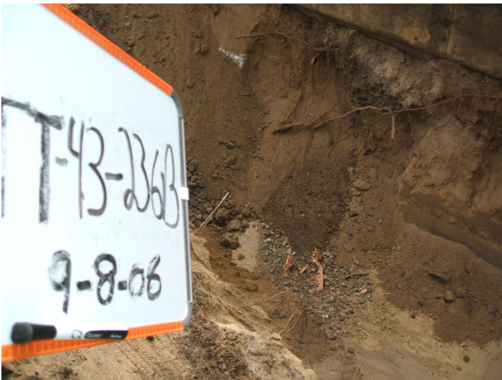
9/8/06: dry well discovered in test trench 43 located on the north side of the building.
