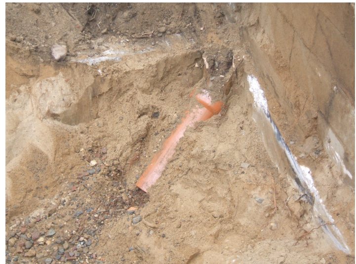
9/8/06: dry well discovered in test trench 45 located on the northwest corner of the building.
