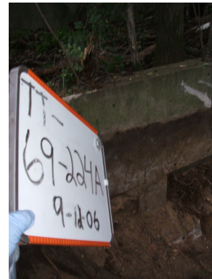
9/12/06 building footing along test trench 69 located on the central portion of the north building wall.
