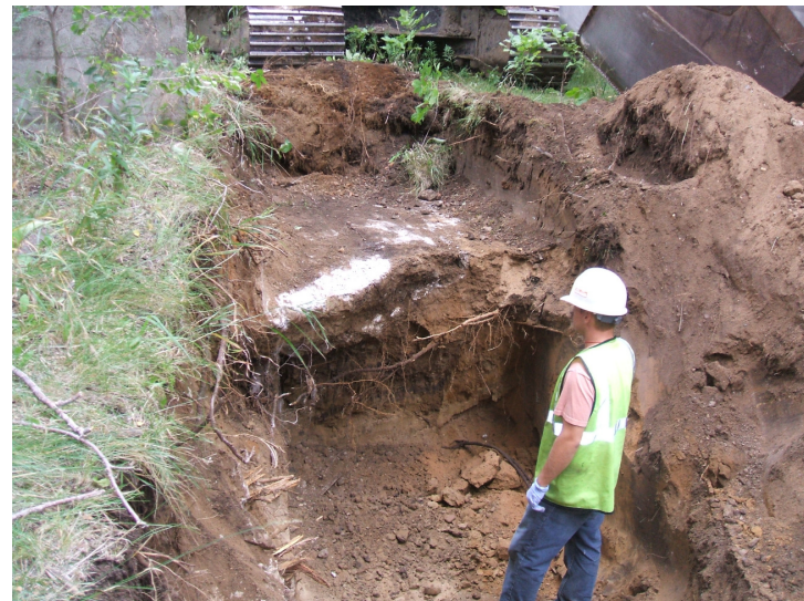
9/8/06: concrete chase for petroleum supply pipes in test trench 49 located along the central portion of the west building wall.
