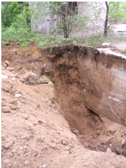
9/8/06: building footing along test trench 49 located along the central portion of the west building wall.
