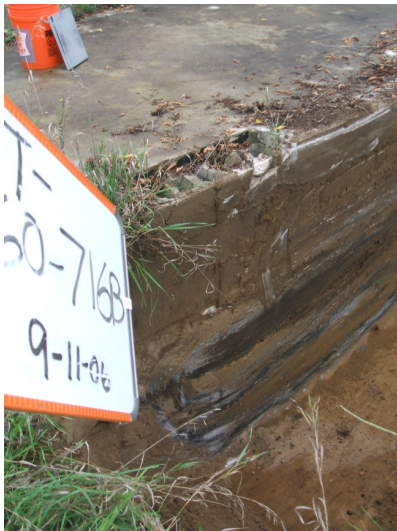
9/11/06: building footing along test trench 60 located on the southwest corner of the building.
