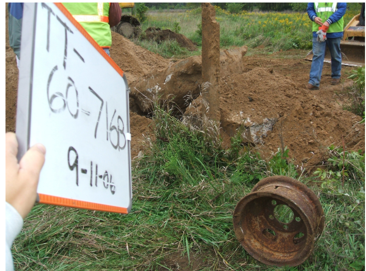
9/11/06: debris excavation from test trench 60 located on the southwest corner of the building.
