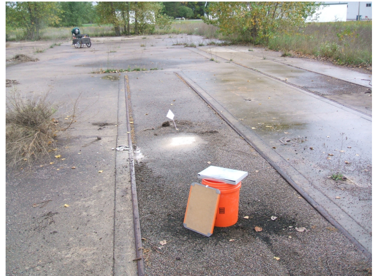
9/11/06: facing west, concrete sample 81 (close) and concrete sample 82 (far) on the concrete building pad.
