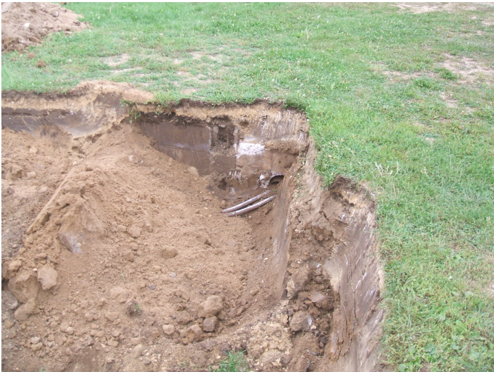
9/11/06: pipes discovered in test trench 59 (building number in photo is wrong) located on the northwest corner of the former building.
